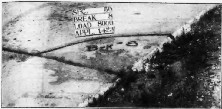
FIG. 18.—TYPICAL CORNER BREAK IN A CONCRETE SECTION.
