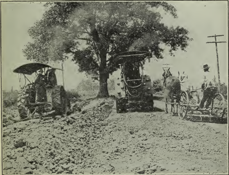
Fig. 6. Grading and Compacting on Earth Road Prior to Oiling. It is Important That an Earth Road Have a Proper Grade and be Thoroughly Compacted Before the Oil is applied.
