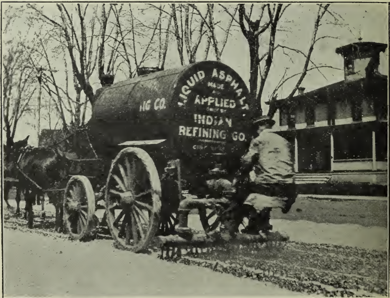
Fig. 18. Applying Oil From a Gravity Distributor. With Such Equipment it is Almost Impossible to Distribute the Oil Uniformly. A Uniform Distribution of the Oil Insures the Best Results.
