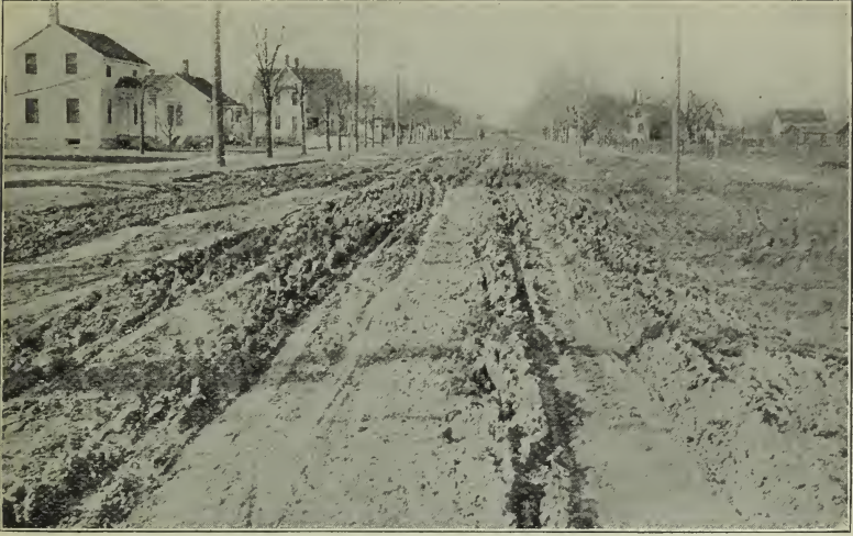
Fig. 5. Proper Drainage is Important on All Earth Roads Before Oiling. There Are Many Flat, Seepy Places That Should be Drained by Tiling. A Line of Tile on Some Sections of Road Will Relieve the Underground Water Pressure and Tend to Prevent the Oil Soaked Earth Crust From Rutting.
