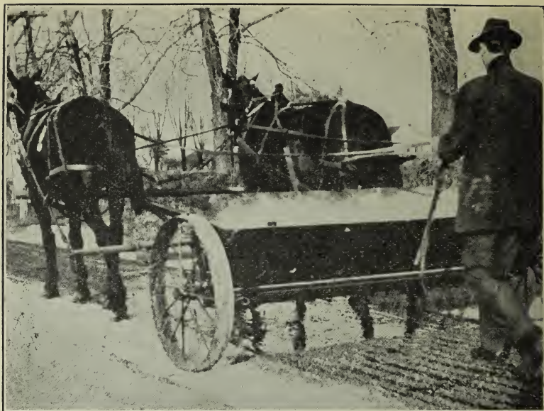
Fig. 25. Sand Spreader Sprinkling Coarse Sand Over Freshly Oiled Surface. The Spreader Holds About One Ton of Coarse Sand or Stone Chips and Drills it Uniformly Over the Oiled Surface. The Spreader May be Loaded From Piles Alongside of the Road or Direct From Wagons. On Light Oils the Spreader May be Hitched to the Sand Wagons and Materials Shoveled Into the Spreader Direct.
