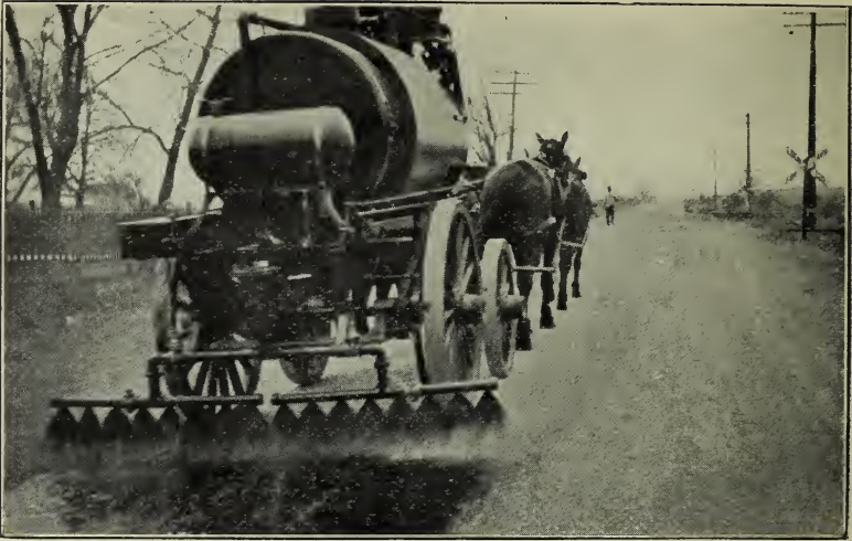
Fig. 17. Applying Heavy Asphaltic Material at the Rate of One-fourth Gallon Per Square Yard of Surface. Material is Heated by Kerosene Burners Beneath the Tank. Note Uniform Distribution of the Asphalt.
