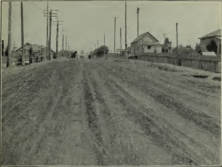
Fig. 3. Oiled Earth Road in California Under Heavy Traffic. Note That the Surface is Rather Badly Rutted.
