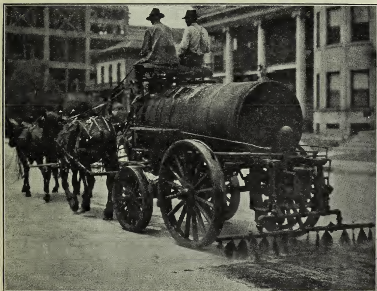
Fig. 16. Pressure Distributor Applying Cold Oil. Poor Results May be Expected From Such Uneven Distribution of the Oil. Note That Only About One-half of the Nozzles Are Working Properly.
