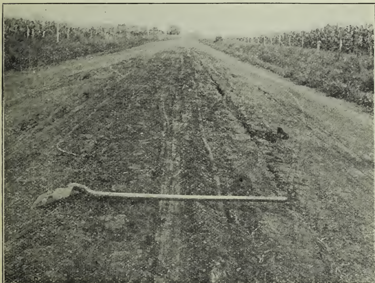
Fig. 24. Oiled Earth Road After Thoroughly Mixing Oil With Top Five Inches of Earth. Three Gallons of Oil Used Per Square Yard of Surface. Condition Not Entirely Satisfactory as it Breaks Up in Winter and Spring. More Economic Results May Be Secured From Continued Surface Oiling.
